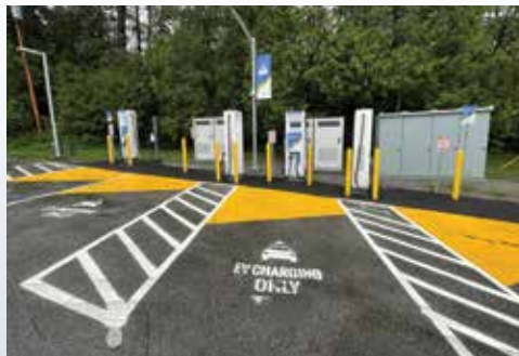
EVOlve NY electric vehicle charging station in Schroon Lake, Essex County
