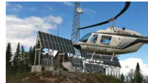
A helicopter accesses a remote, off-grid radio communications network site in Maine
