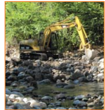
Ongoing restoration of Johns Brook, Keene Valley, NY, September 2013. Photo courtesy of Ausable River Association
